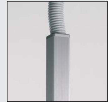
Cables are led into the ceiling construction inside a flexible tube.
