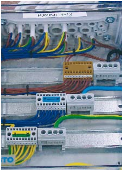
A typical application for screwless terminals: tapping of neutral earth and live conductors.
