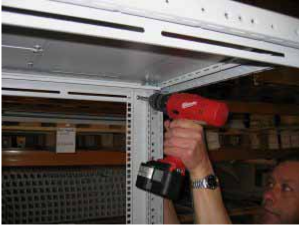
5. Fasten 19" rails in each end by placing klipnut in slide of bearing. Screw in screws into top- and bottom.
